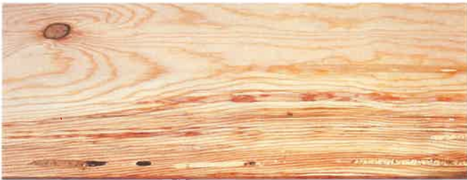
Figure 11-13. Peck is caused by fungus. Grub holes are caused by insects. (Western Wood Products Assoc.)
