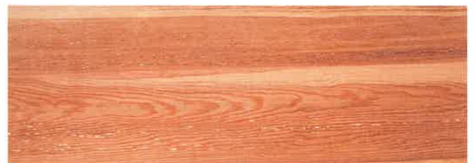
Figure 11-17. Honeycomb is caused by separation of wood rays. Top—It is seen as voids in the end of cut lumber. (Forest Products Laboratory) Bottom—Honeycomb as depressions in surfaced lumber. (Western Wood Products Assoc.)
